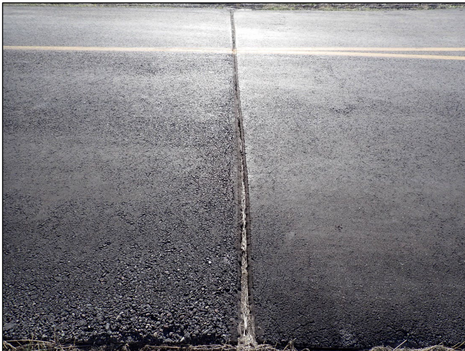
TW-02-04: L&T Cracking
