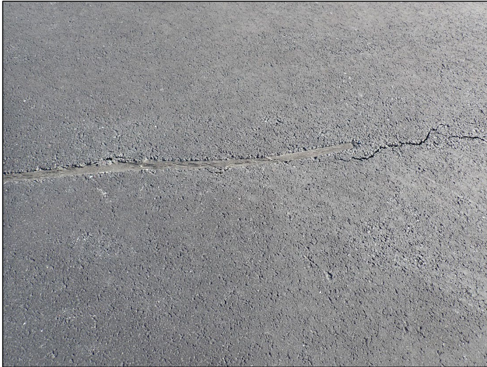
AP-01-05: L&T Cracking
