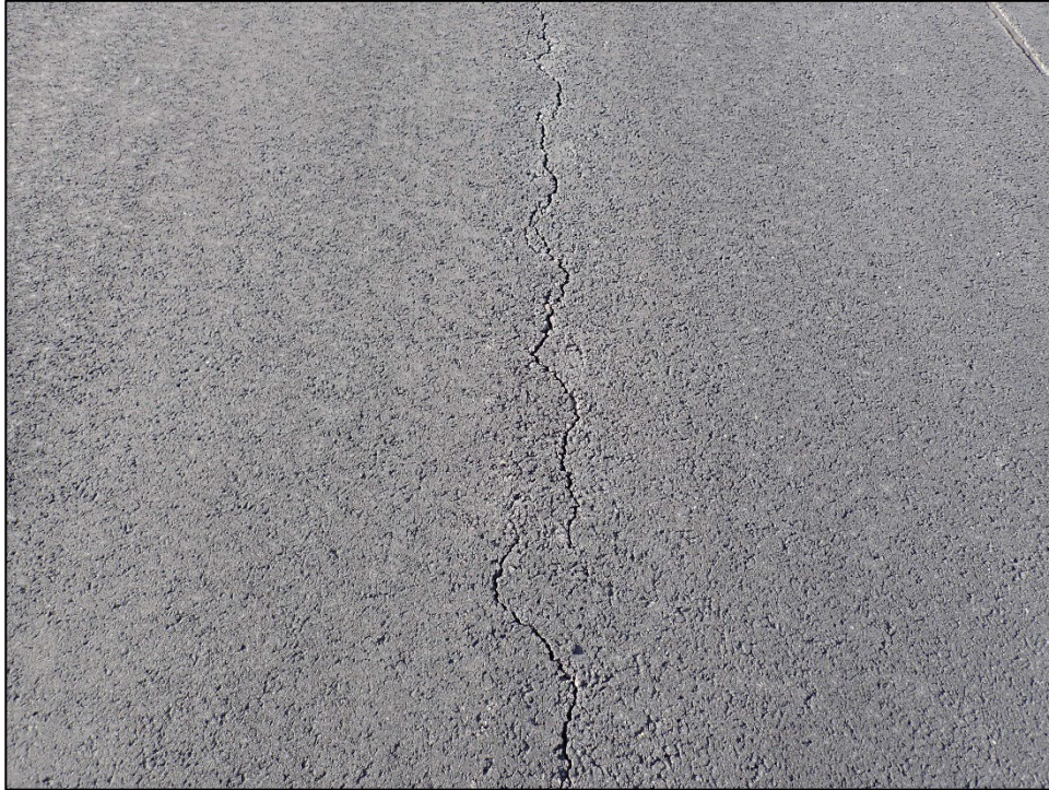
RW13-01-21: L&T Cracking
